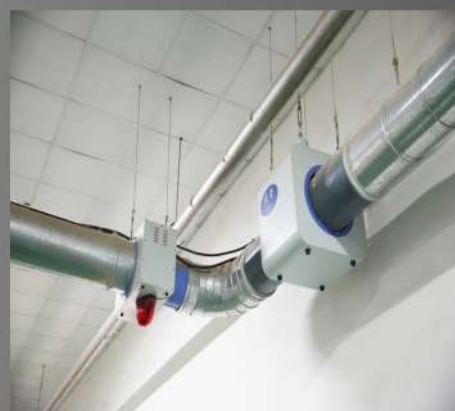
MULTY DUST FILTRING UNIT
